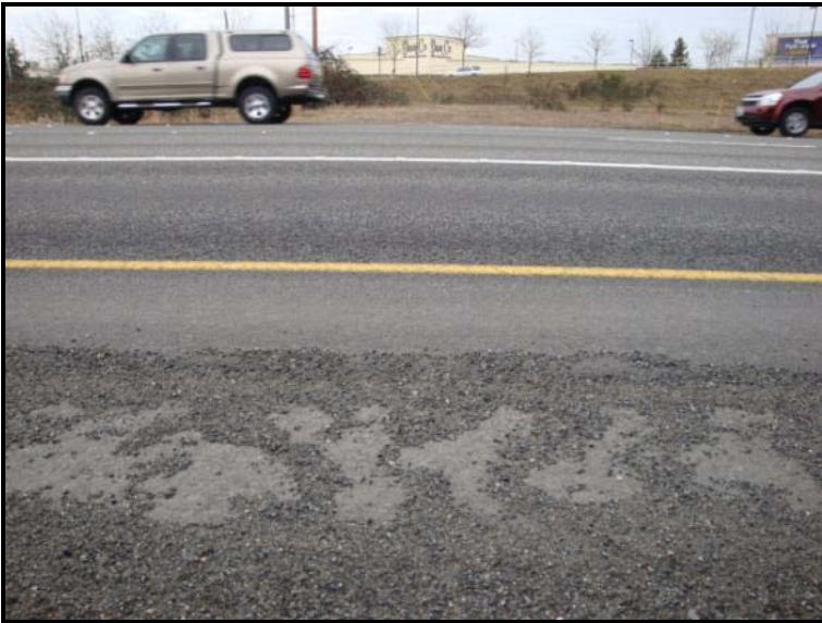
Pavement raveling on I-5 OGFC-AR test section two years after install.
