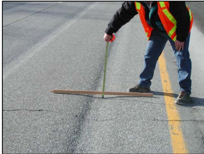
Rutted section of pavement installed in the 1990's.
